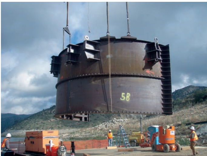
Lifting units 5 and 6 to a FlexiFloat barge and subsequently transported to the dam.
