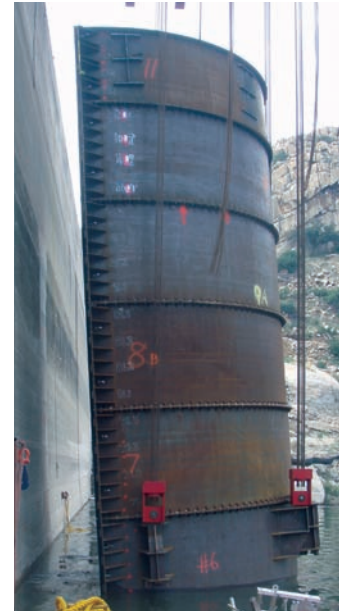
Attachment of units 1-11 to the face of the dam. The cofferdam is tilted to fit the slope of the concrete face before being lowered to the required elevation.
