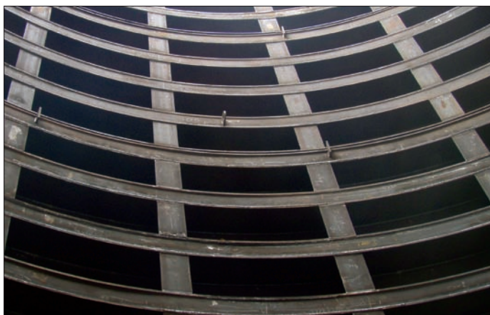
Inside view of the complex shell construction necessary to withstand the loads while the cofferdam is dewatered.
